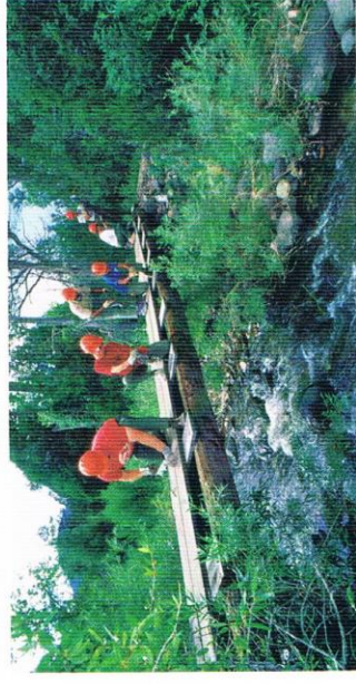
These Scouts repair a footbridge across a mountain stream. Conservation work became even more visible with the launching of Scouting's Project SOAR (Save Our American Resources) in 1970.
