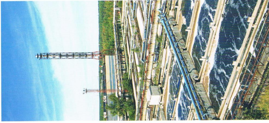
Water treatment facility
